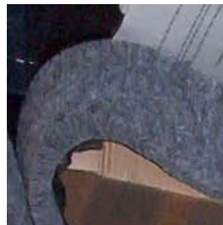
Figure 9. Insulation material behind the chilled ceiling panels
